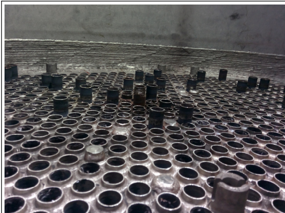
Figure 13: tubes protruding upside
